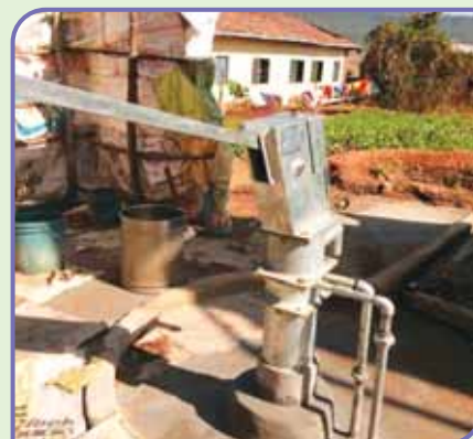
Solar Handpumps, Jashpur
